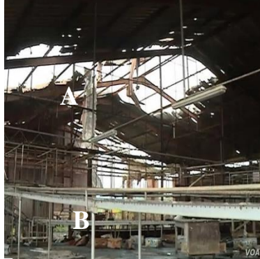
Photo 2: A Burned Rubber Factory in Mafanja-Tiko Source: Authors, August 2020
