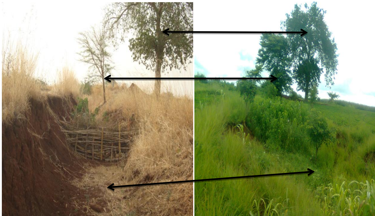
Figure 8: Shows the difference between before and after gully rehabilitation the same site
